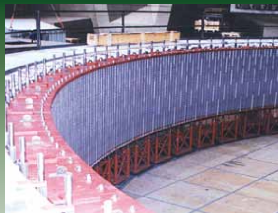
144 Screw and Cap assemblies support the outer wall of a large generator assembly at the Grand Coulee Dam.
